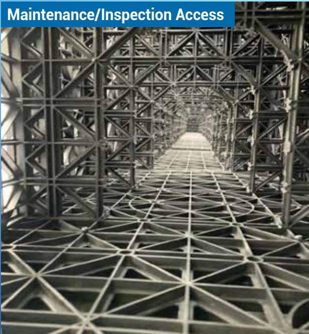
150m 3 OSD Tank Under Carpark
